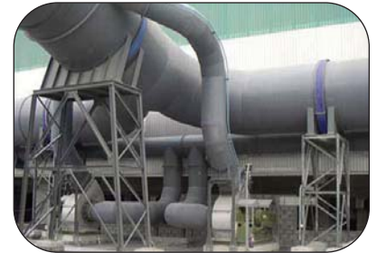
Aluminum smelter potroom off-gas ducting system with Thorburn Flexi-Duct™ expansion joints installed
