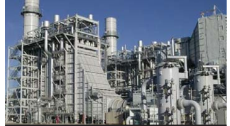
Clean Power Generation
