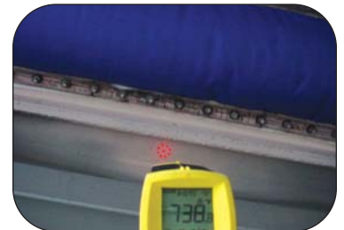
Thorburn's Site team measuring the temperature of an expansion joint's mating structure in an HRSG in Kansas, USA
