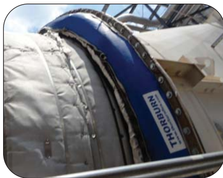
Gas turbine exhaust expansion joint with Thorburn's KLFC GSM installed
