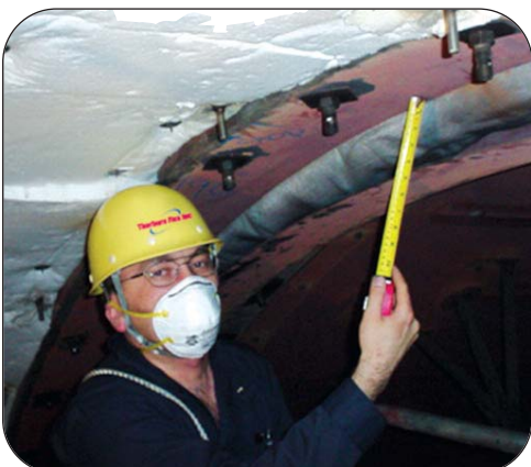
Thorburn's engineer examining the ash barrier inside a large diameter HRSG inlet expansion joint with a 150mm offset opening at a Singapore power plant
