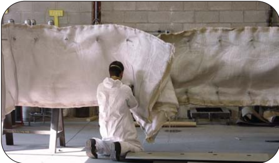
Thorburn's technician in South Africa installing a cavity pillow on a Flexi-Duct™ inlet HRSG expansion joint
