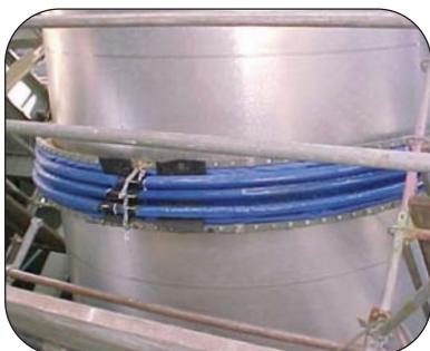
Thorburn's Barrel Hoop expansion joints installed on the primary air lines at the JEA CFB Power Station in Florida
