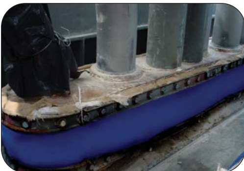
Six non-insulated steam pipes grouped into one Thorburn Flexi-Duct™ penetration seal expansion joint at a Florida power plant
