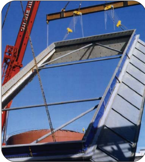
Thorburn's outlet expansion joint being installed at an HRSG in Huntstown, Ireland
