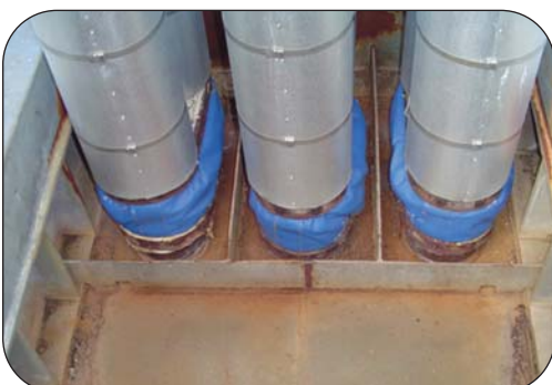
A series of fully insulated dual steam pipes into one Thorburn Flexi-Duct™ penetration seal expansion joint in a Mexican power plant
