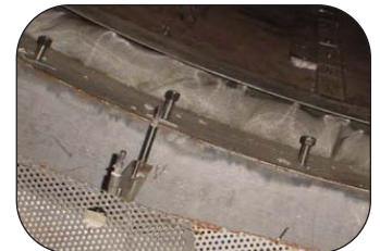
Thorburn's gas turbine expansion joint before turbine washing showing packed thermal insulation
