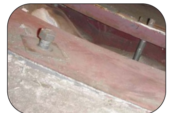
Thorburn's gas turbine expansion joint after turbine washing showing compacted insulation creating a cavity
