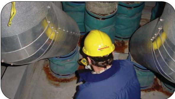
Thorburn's technician recording temperature of a penetration seal at an HRSG in Oregon, USA
