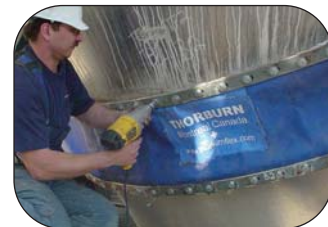
Thorburn's technician providing on-site training at a CFB power plant in Jacksonville Florida USA
