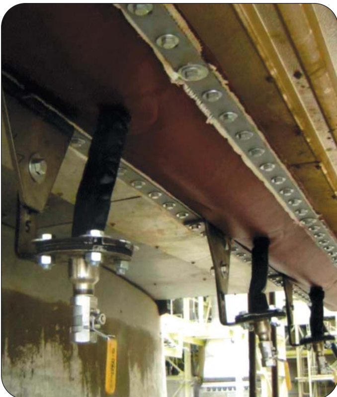
Thorburn's M12 GSM with integral drains on the bottom of a rectangular Flexi-Duct™ expansion joint complete with flex hoses and ball valves at an Egyptian power plant
